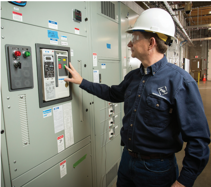
Smart Grid Project Manager Kevin Whitener at the low voltage switchboard in the Salem Smart Power Center.
