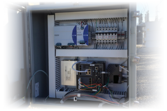
Turnkey substation communications enclosure designed, built, and tested by Eaton
