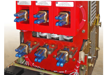
All New Power Conductors
