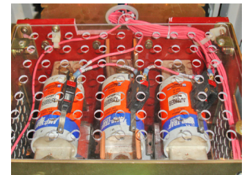
Easily Accessible Fuses
