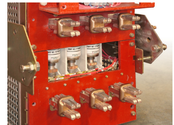
All New Power Conductors
