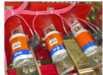
Easily Accessible Fuses
