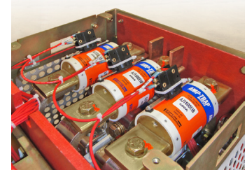
Easily Accessible Fuses
