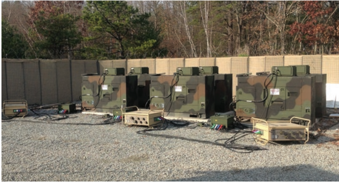
Figure 2: Eaton Intelligent Mobile Power Distribution System
