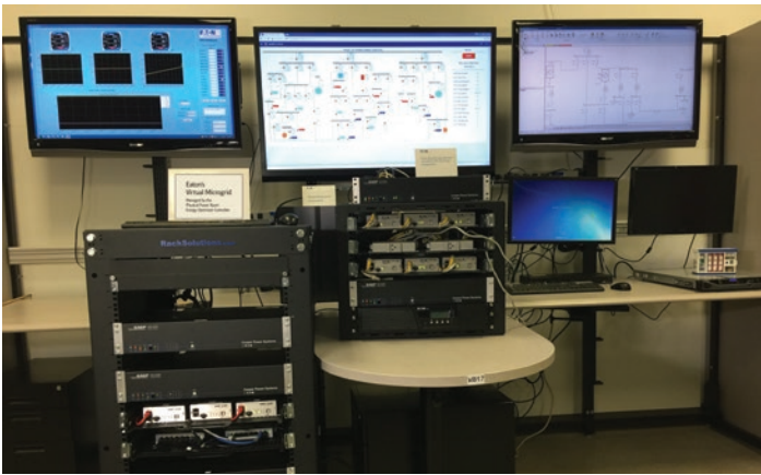
Figure 6: Eaton’s virtual microgrid managed by the physical Power Xpert Energy Optimizer™ controller
