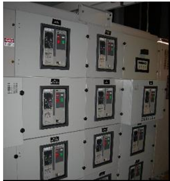
Figure 5. Retrofilled Fuses with Breakers Example
