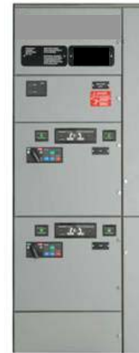
Figure 17. New "Safety-by-Design" Motor Control Center
