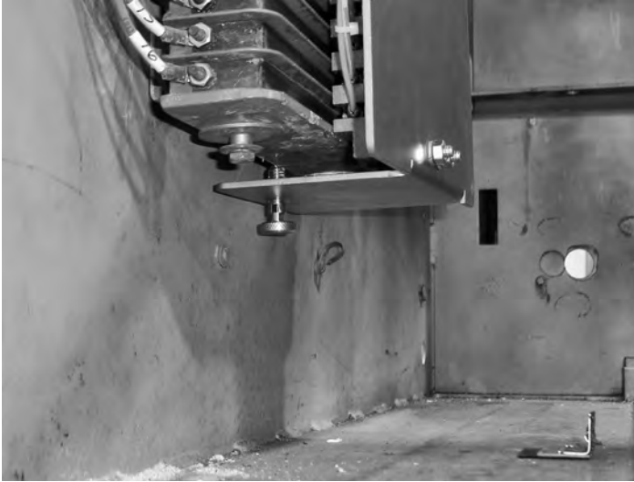
Figure B.5. Test Jumper Installed on Circuit Breaker
