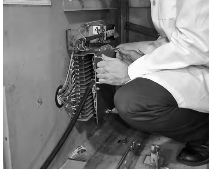
Figure B.8. Test Jumper Installed on Circuit Breaker
