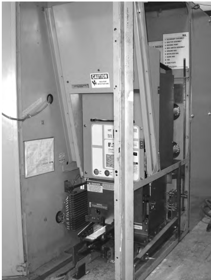
Figure 5.12. Circuit Breaker in the 'Connect' Position
