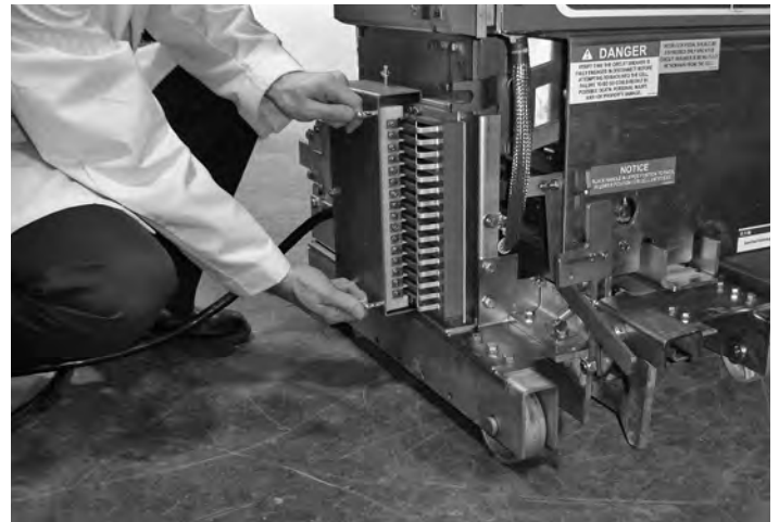
Figure B.9. Test Jumper Installed on Circuit Breaker
