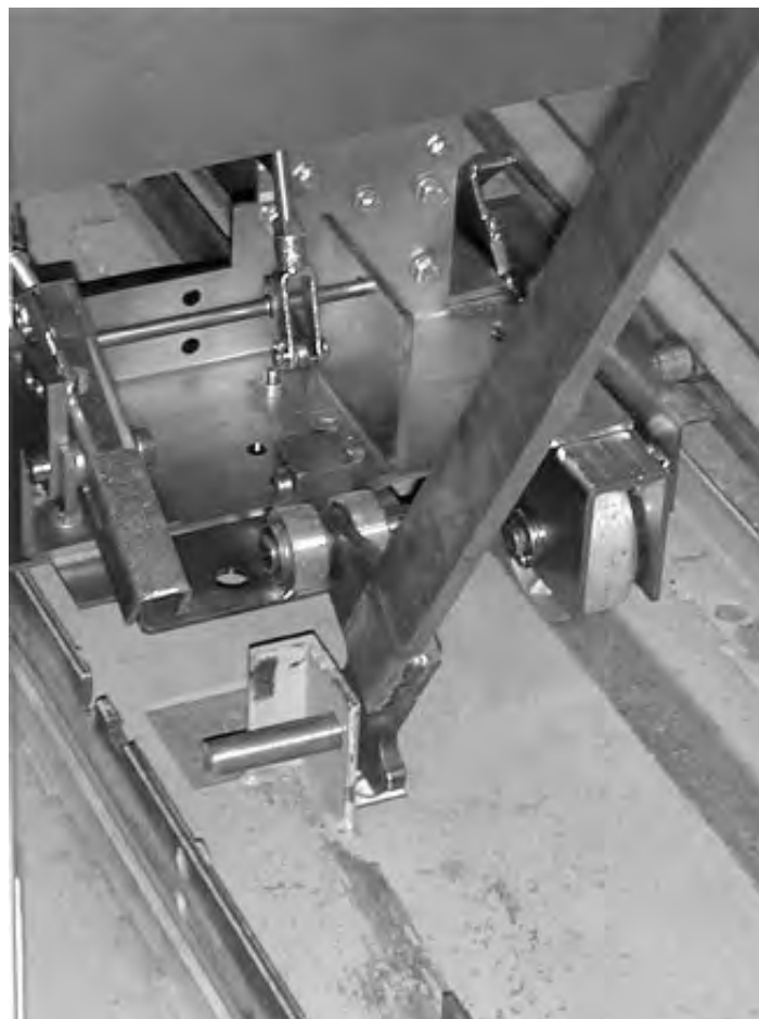
Figure A.1. Rack-In Position of Levering Handle
