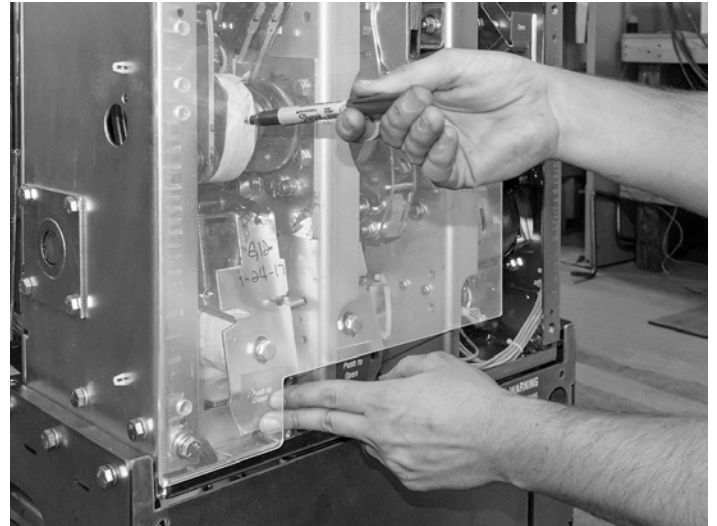
Figure 6.8. With Marker in Hole "C", While Closing Circuit Breaker
