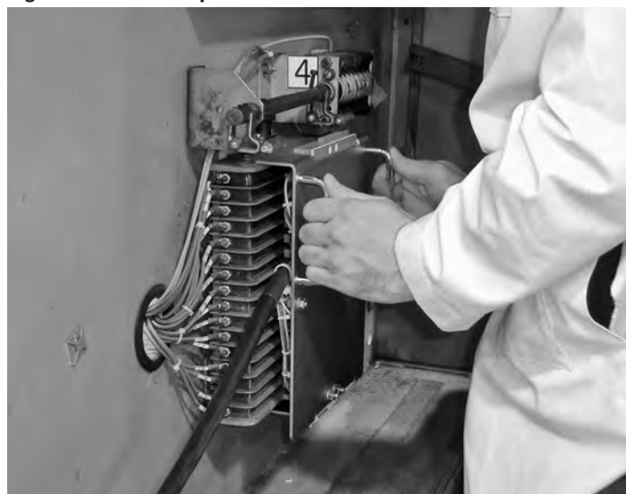
Figure B.4. Test Jumper Installed on Circuit Breaker
