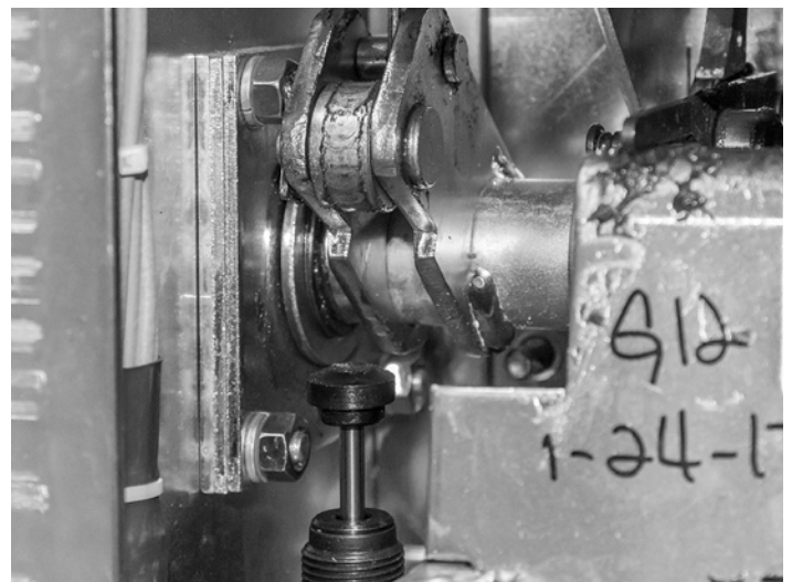
Figure 6.9. Pole Shaft Located On Left Side Of Circuit Breaker
