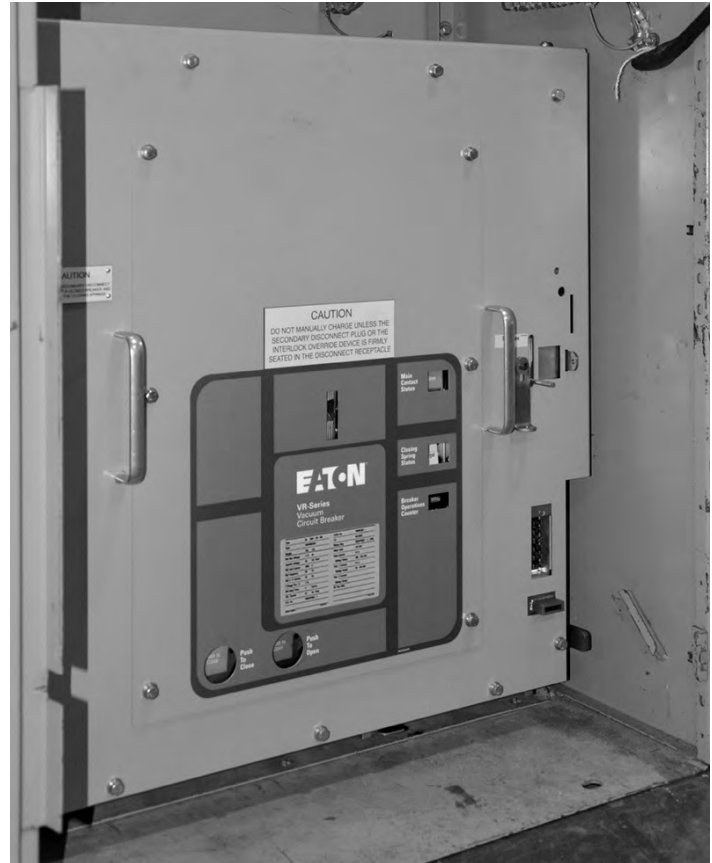
Figure 5.5. Disconnect Position (15PV-VR 1200A Shown)
