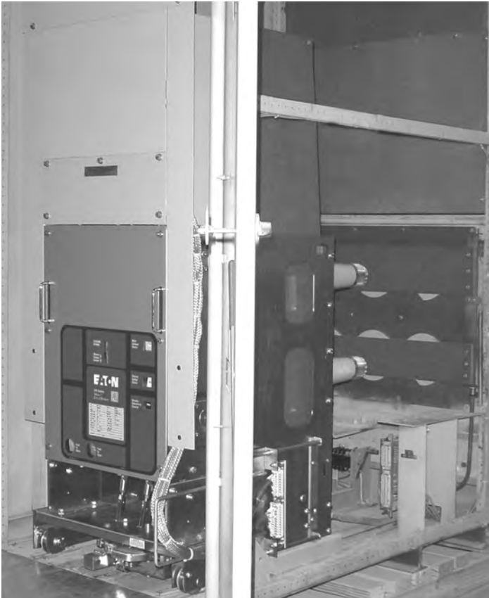
Figure 5.2. DST-2-75-VR in the Disconnect Position
