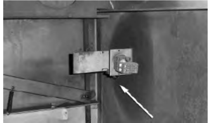
Figure 4.4. Cell TOC Switch
