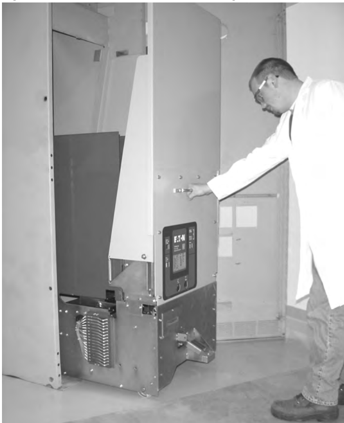
Figure 5.11. FC-VR Withdrawn From Switchgear
