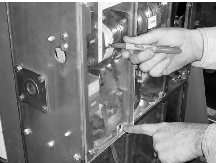
Figure 6.10. With Marker in Hole "C", While Closing Breaker
