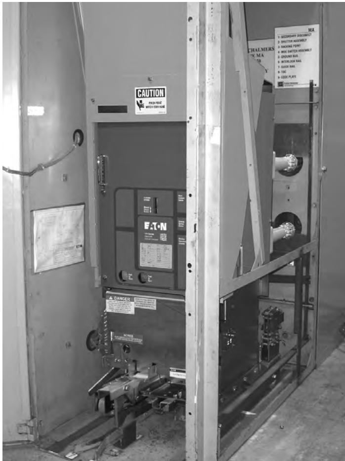
Figure 5.10. Circuit Breaker in the Test Position
