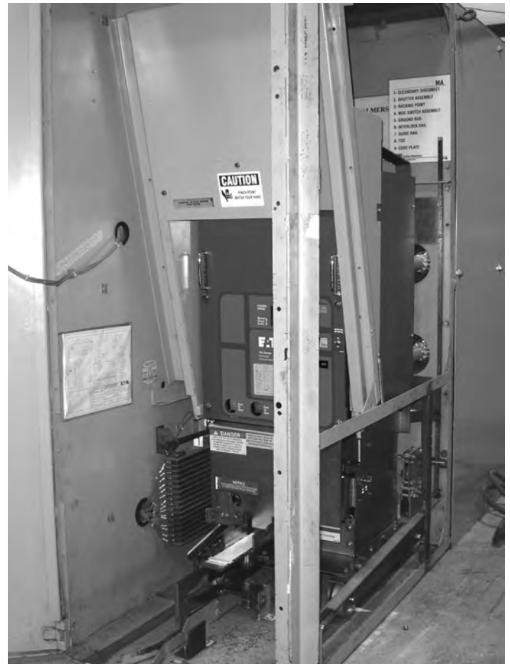
Figure 5.12. Circuit Breaker in the Connect Position
