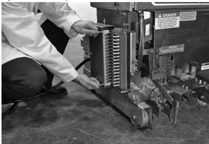
Figure B.9. Test Jumper Installed on Circuit Breaker
