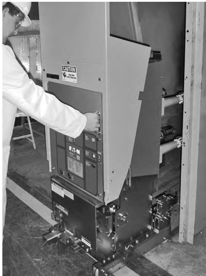
Figure 5.9. Circuit Breaker in the Withdrawn Position
