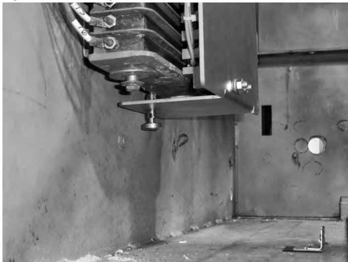
Figure B.5. Test Jumper Installed on Circuit Breaker
