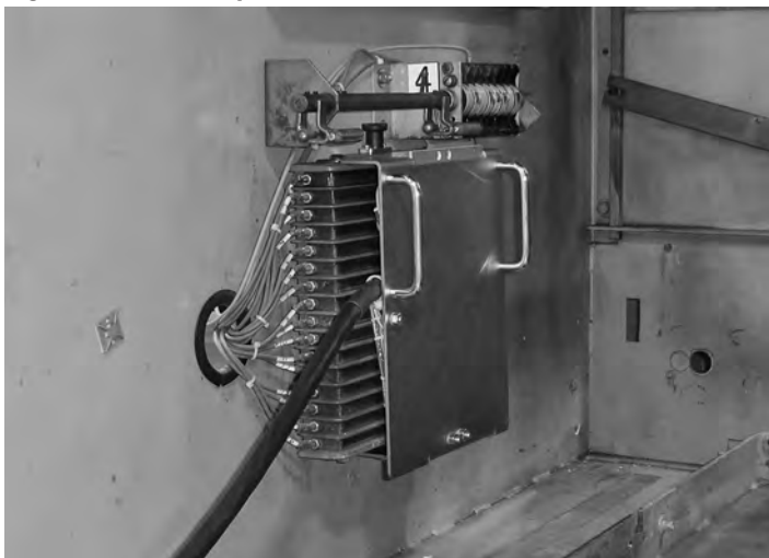
Figure B.7. Test Jumper Installed on Circuit Breaker
