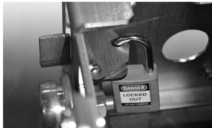
Figure 5.2. Lock-Out Provision (Viewed Inside Breaker Frame)
