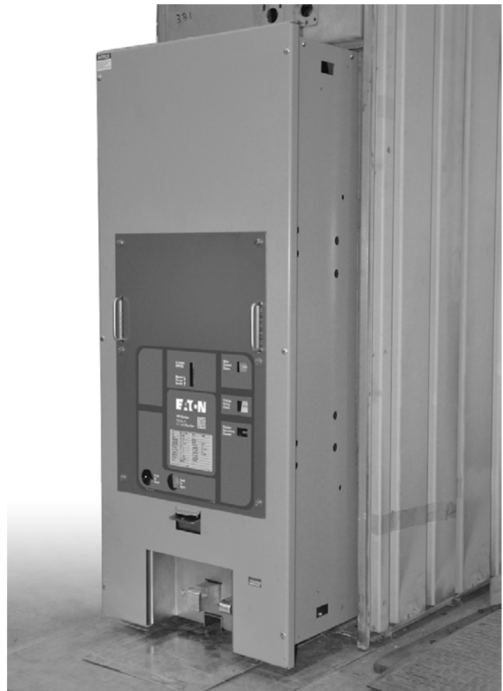
Figure 5.2. AMH-VR in the Disconnect Position
