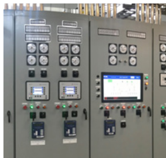
Paralleling switchgear control station
