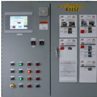
Control panel closed
