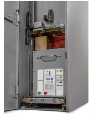
VHC breaker installed
