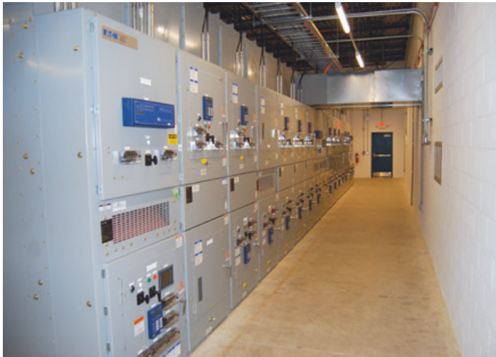
Block building containing switchgear
