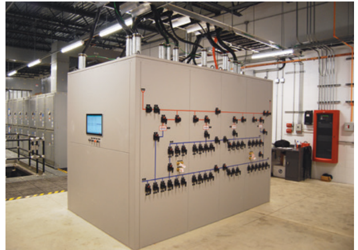
Duplex control board complete with HMI, control switches and 69kV relays (on opposite side, not shown)
