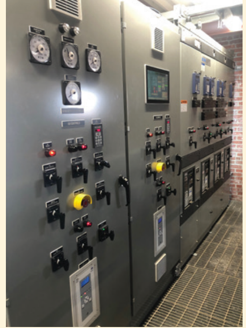
Control system interface
