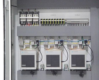
Motor Control Panels with 3 Phase Disconnect
