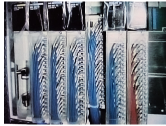
PLC and Motor Control Panels
