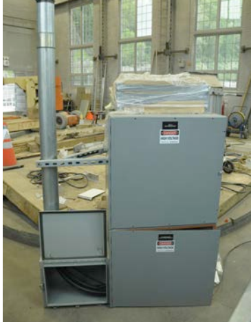
Combination generator termination cabinet (surge equipment) and high-resistance ground enclosure (hydroelectric facility in West Virginia)
