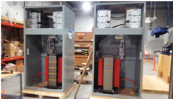
Two high-resistance ground cabinets (hydroelectric facility in Virginia)
