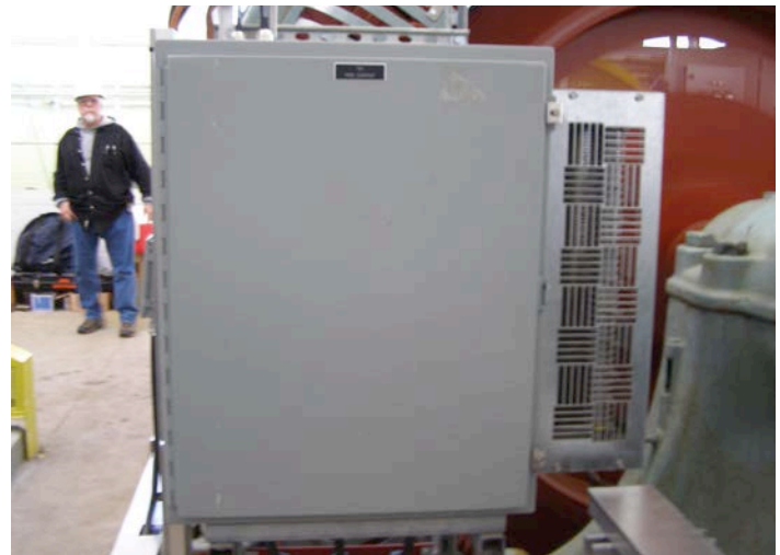
Small hydro high-resistance ground and generator neutral enclosure (hydroelectric facility in Maine)
