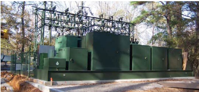
New Eaton modular integrated transportable substation (MITS) in front of open air substation to be retired shown behind.
