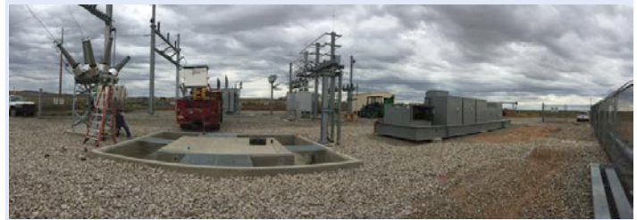
Jemez Mountains Electric Cooperative: installation of pad to house new transformer, new breaker installation, and MITS shown on right.
