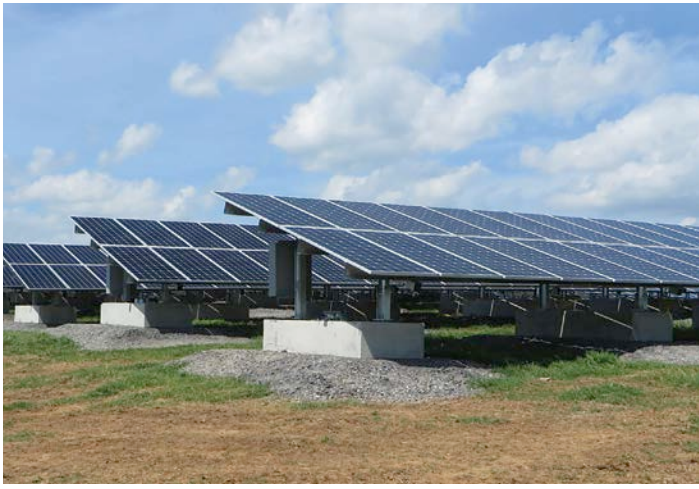
Concrete ballasted ground mount racking system installed on capped landfill
