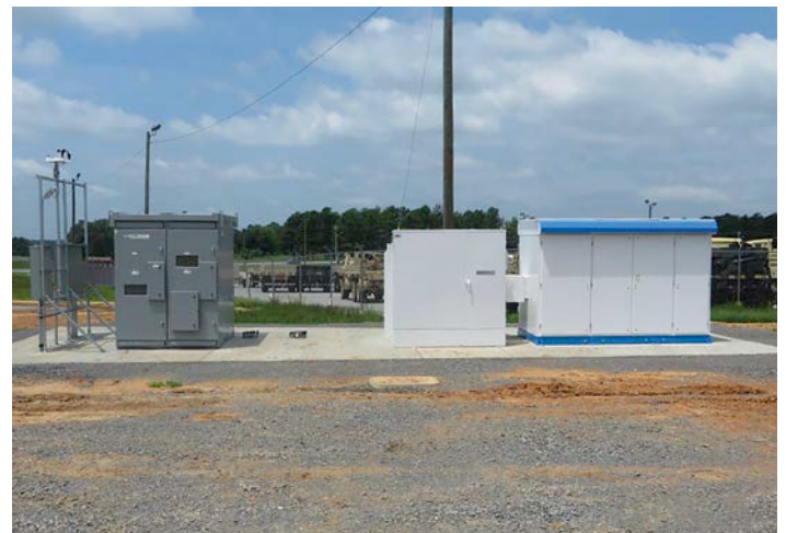
Eaton MV switchgear, Power Systems series MV transformer and Power Xpert solar inverter
