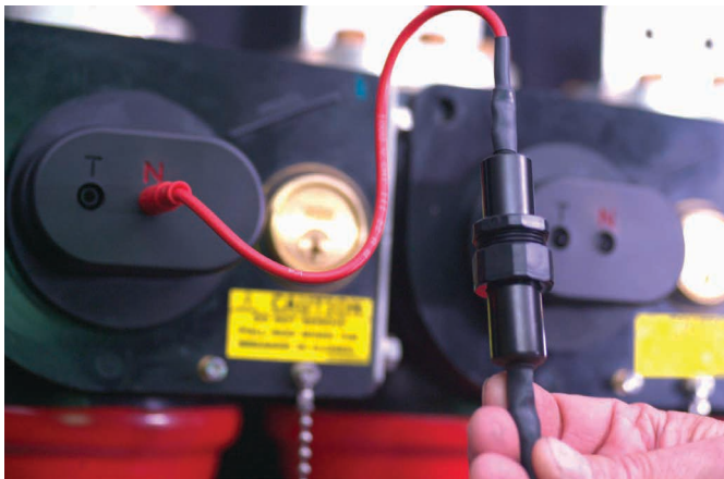
Figure 5 – Test lead used to power test set
