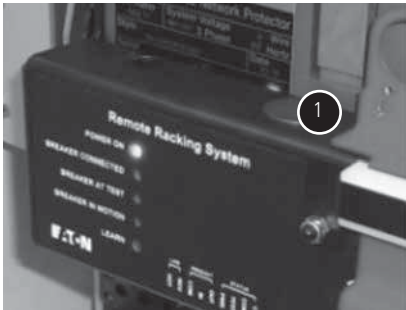
① With unit powered, power on LEDs should be illuminated.
