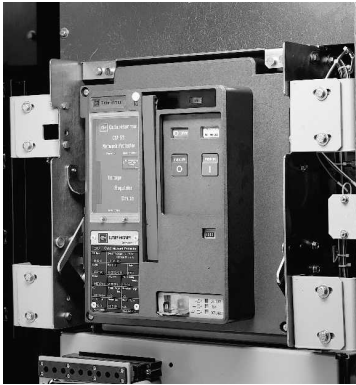
Fig. 8a Breaker in Connect position
