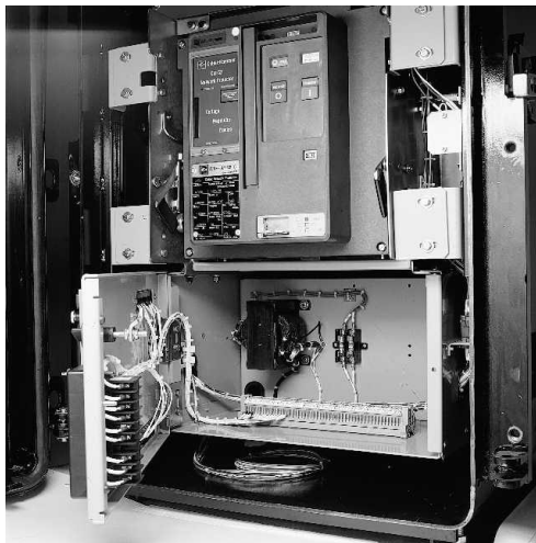
Fig. 6 Relay Module Panel Opened
