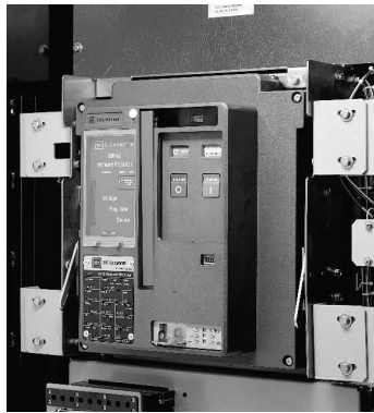
Fig. 8b Breaker in Test position
