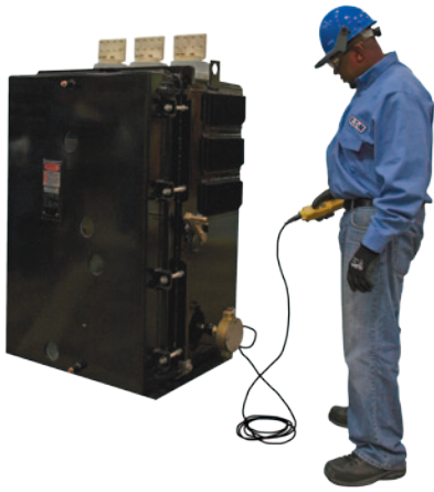
Figure 1. Remote racking unit can be operated by a hand-held pendant.
