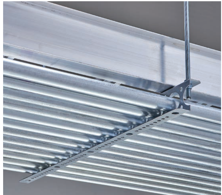
Conduit trapeze support with cable tray
