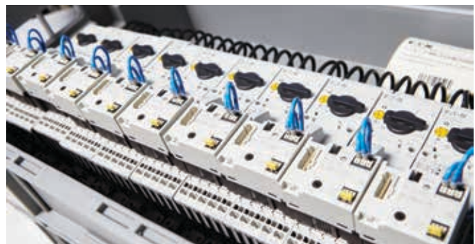
Image 7: The delivery of components in kits supports the processes within the company and also paves the way for lean production.
