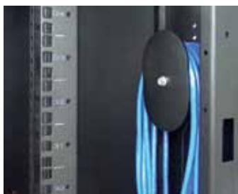
Take-up Spools Efficient and TIA/EIA-568-A compliant organization of excess cabling within the enclosure.
