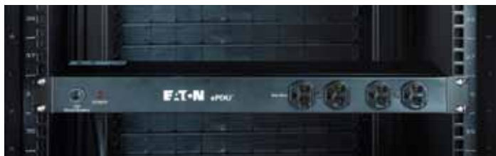
ePDU mounted horizontally in rack
