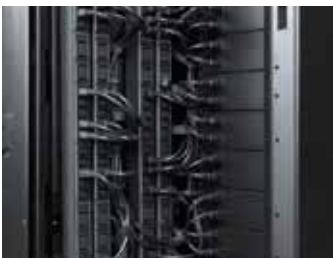
Lacing bars are provided for power and cable management mounting.
