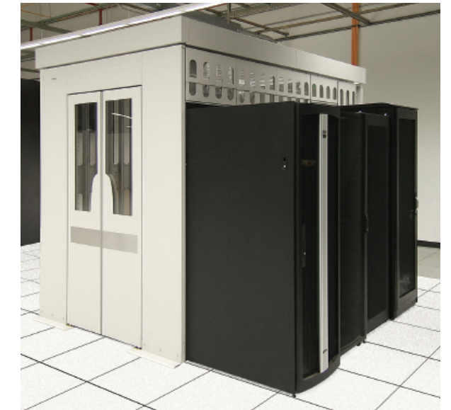
Shown above—ICS featuring End of Row, café-style doors and vertical blanking panels to accommodate third-party enclosures.
