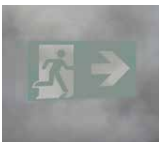
Badly illuminated escape sign
