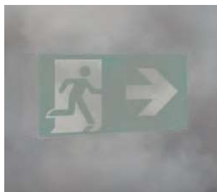
Badly illuminated escape sign
