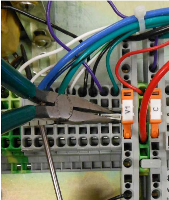
Figure 24. Removing jumper between C2 and C3
