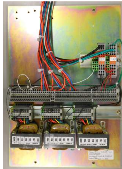
Figure 11. Typical CL-7 control multi-phase back-panel
