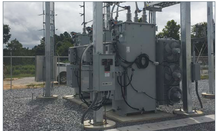
Substation class regulators
