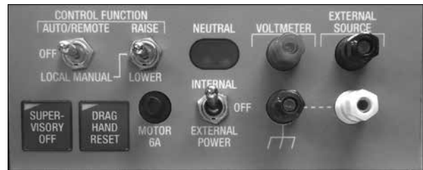
Figure 4. Control panel switches.
