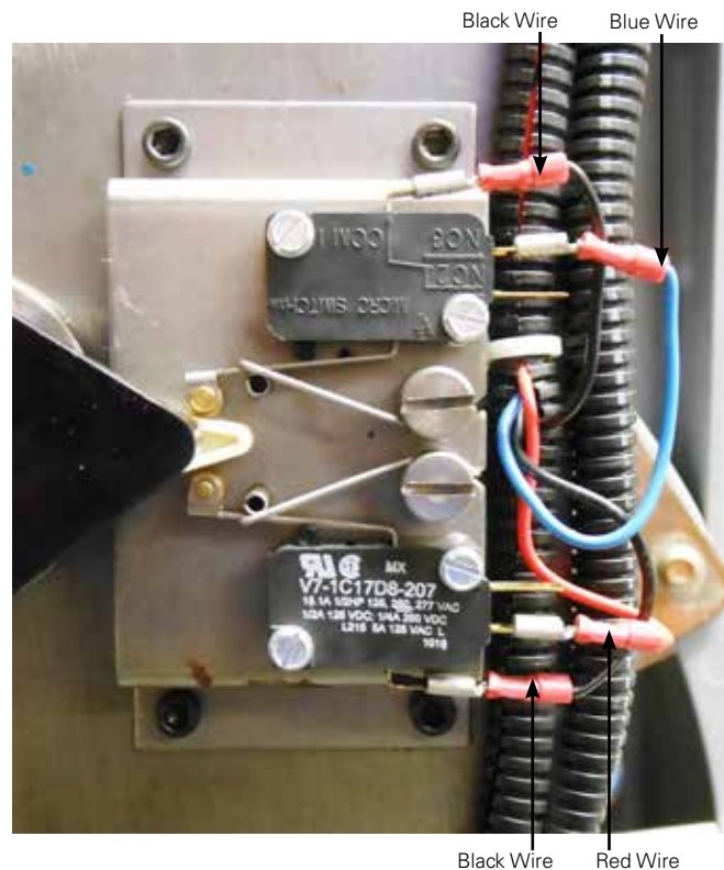
Figure 3. Holding switch on molded polymer-style QD5 tap-changer.
