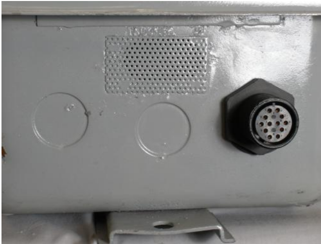
Figure 40. QCA connector coming from the bottom of the General Electric control box.
