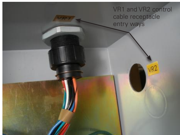
Figure 2. Enclosure entry way examples.
