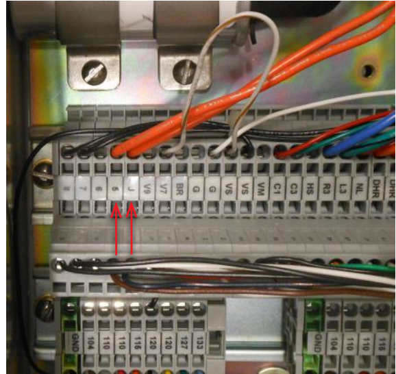
Figure 11. Orange wires shown relocated for VR1 and VR2. Each non-Cooper Power series connected voltage regulator requires relocation of an orange wire.
