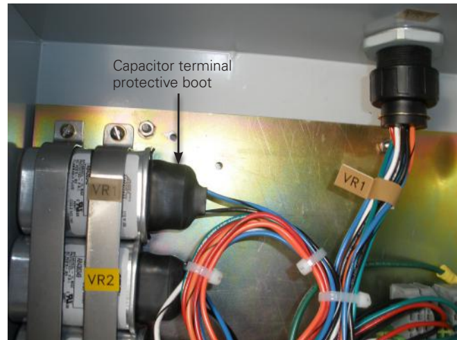
Figure 14. Capacitor protective boots.
