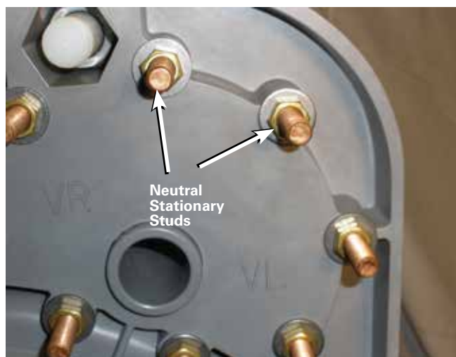
Figure 44. Reinstalling neutral stationary and hardware.
