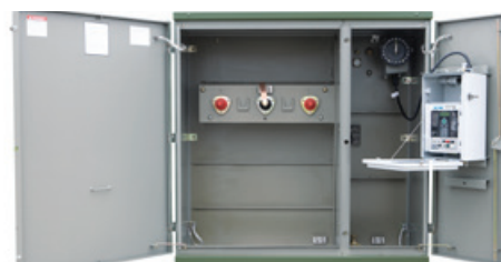
Single-phase pad-mounted regulator with CL-7 control
