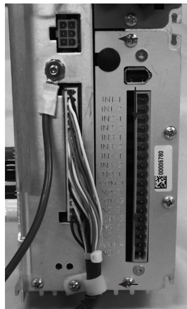
Figure 5. Securing the I/O module with screws into the accessories slot of the main control panel. Note that in this installation, the power cord is not required.
