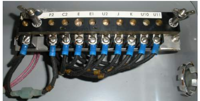
Figure 24. Siemens Corporation enclosure terminal block
