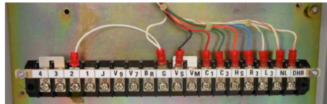
Figure 9. Proper jumper arrangement on 18-position terminal board for the CL-7 voltage regulator control
