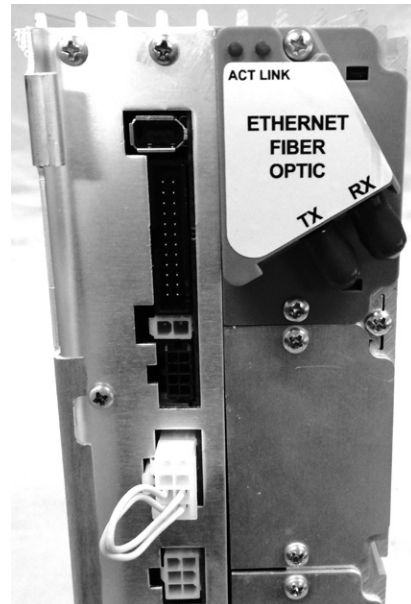
Figure 12. One communications module installed with the other slot covered
