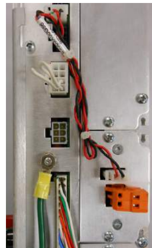
Figure 60. DC power supply (13.5 Vdc) installed in the side of a CL-7 control
