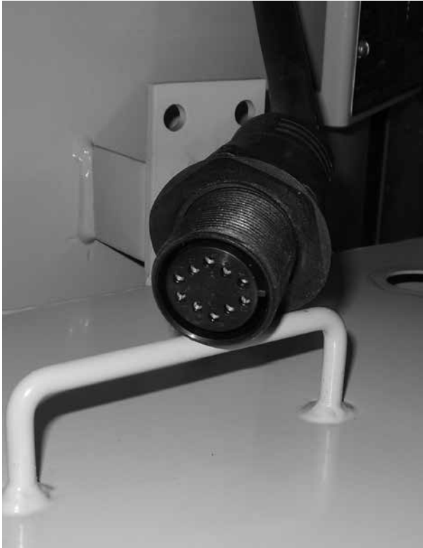
Figure 6. Inspecting the control box end off the quick-disconnect cable
