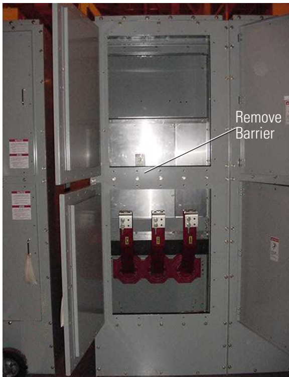
Figure 4. Main Bus Installation with Bus Barriers Installed. Viewed from Rear with Doors Open (Typical 1-High Construction Shown).
