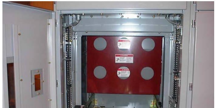
Figure 16. Ring Type CTs with Shutters Closed and CT Barrier in Place.
