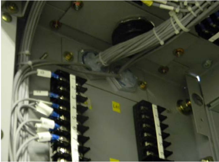
Figure 6A. Caulk Filling Between Low and Medium Voltage Sections.
