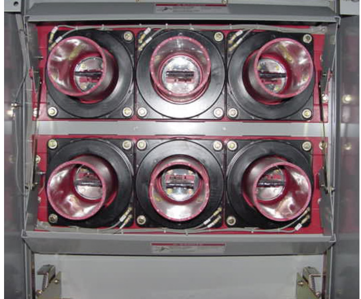
Figure 15. Automatic Shutters - Ring Type CTs with Shutters Open and CT Barrier Removed.
