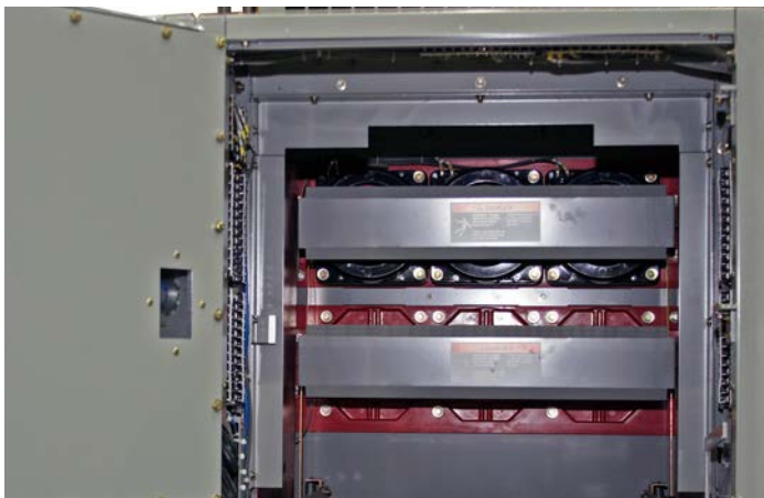
Figure 14. Automatic Shutters - Ring Type CTs with Shutters Closed and CT Barrier Removed
