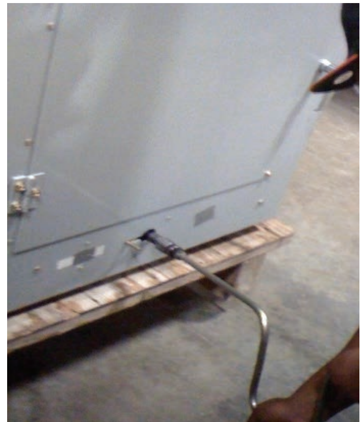
Figure 32. Racking the Breaker/Auxiliary.
