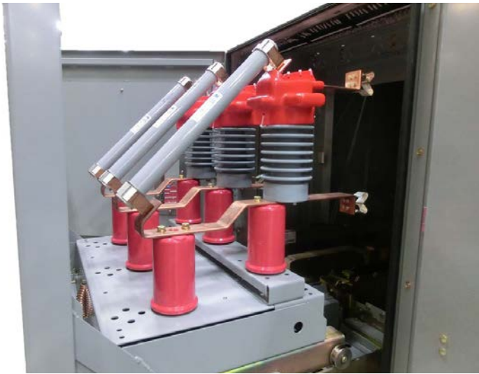
Figure 40. Typical Fuse Drawer Drawn Out onto Extension Rails.
