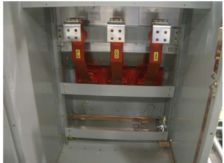
Figure 3. Ground Bus Installation.
