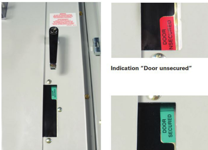
"Door Secured" and arc-resistant
