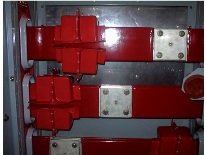
Figure 5. Main Bus Installation with Bus Barriers Removed.
