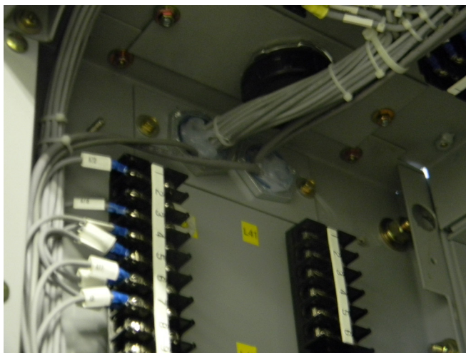
Figure 5. Caulk Filling Between Low and Medium Voltage Sections.
