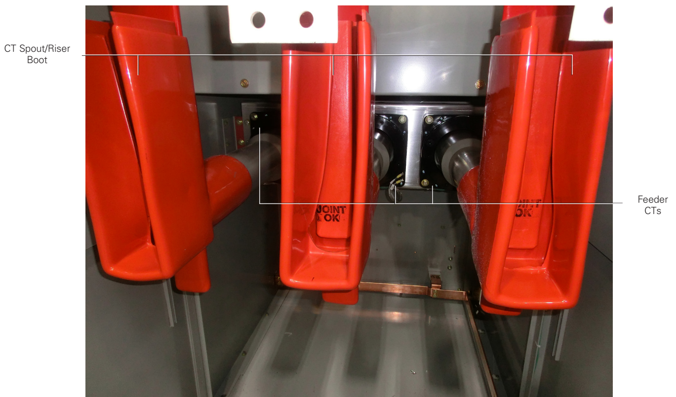
Figure 7. Assembled Switchgear (Shown with Rear Doors Opened).
