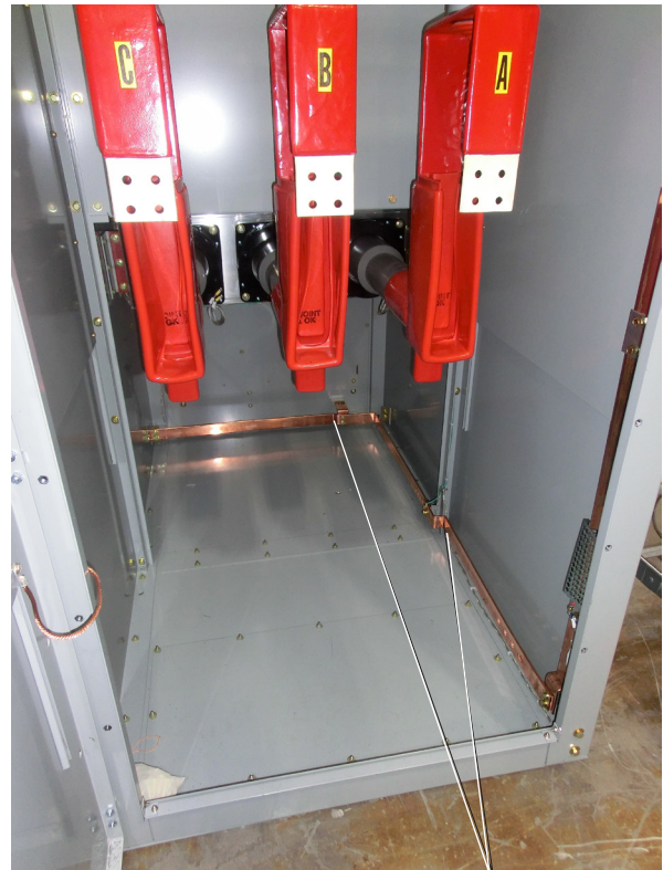
Ground Bus (Rear View)
