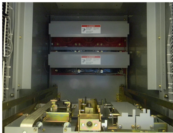
Figure 10. Breaker Primary Disconnect Shutters (CT Barrier Removed).
