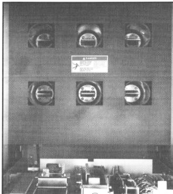
Figure 9. CT Barrier (Shutters Blocked Open).
