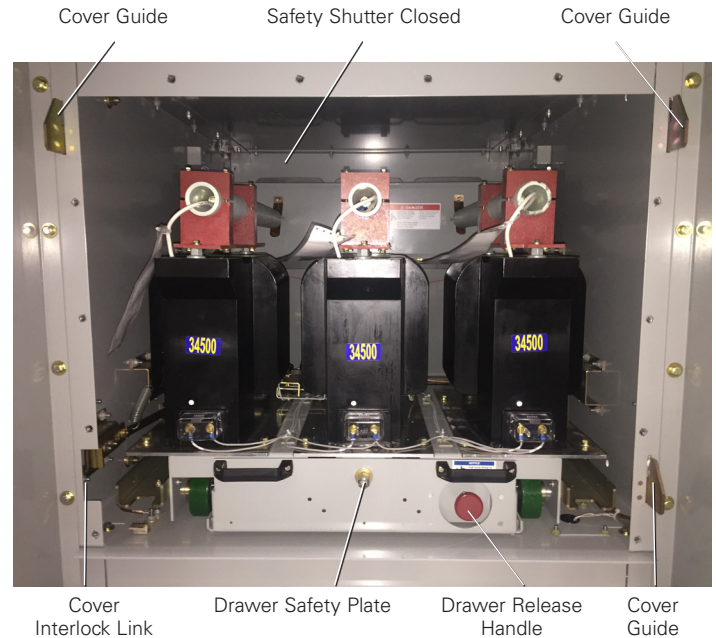
Figure 7. Auxiliary Compartment with Cover Removed and Drawer in the Disconnect Position.
