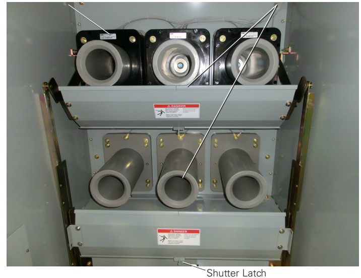
Figure 11. Breaker Compartment with Shutters Latched Open.
