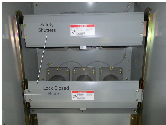
Figure 10. Breaker Compartment with Shutters Closed.
