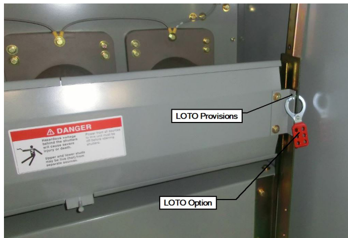
Figure 12. Lockout-Tagout Provision for Shutter LOTO.
