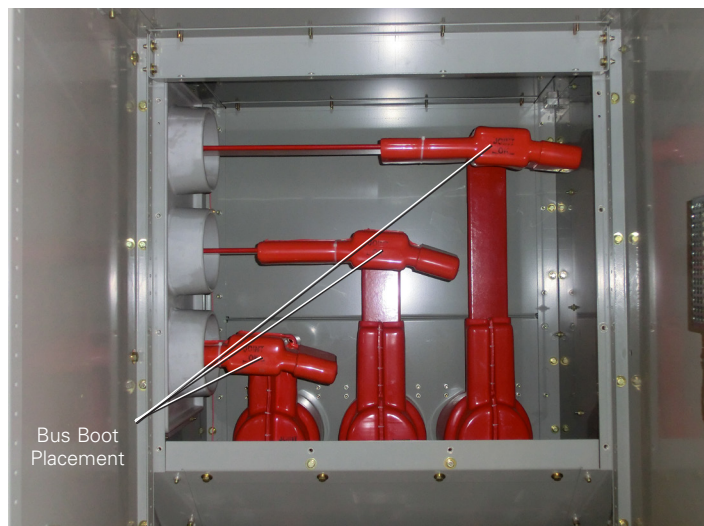
Figure 5. Main Bus Installation – Barriers Removed Showing the Bus Joing Insulating Boots.
