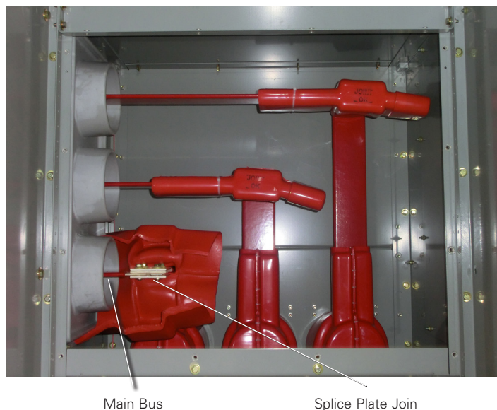
Figure 4. Main Bus Installation – Barriers Removed Showing the Main Bus Connections.
